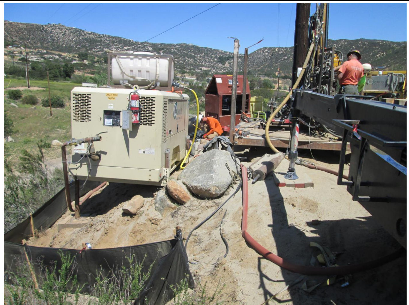
Photo 2: In accordance with APM-HYD-1 and the Project SWPPP, silt fencing installed around work areas was observed in good condition and functional. In accordance with APM-HAZ-2 and the Project Fire Plan, fire safety equipment was staged on site and a fire extinguisher was mounted on the compressor.
