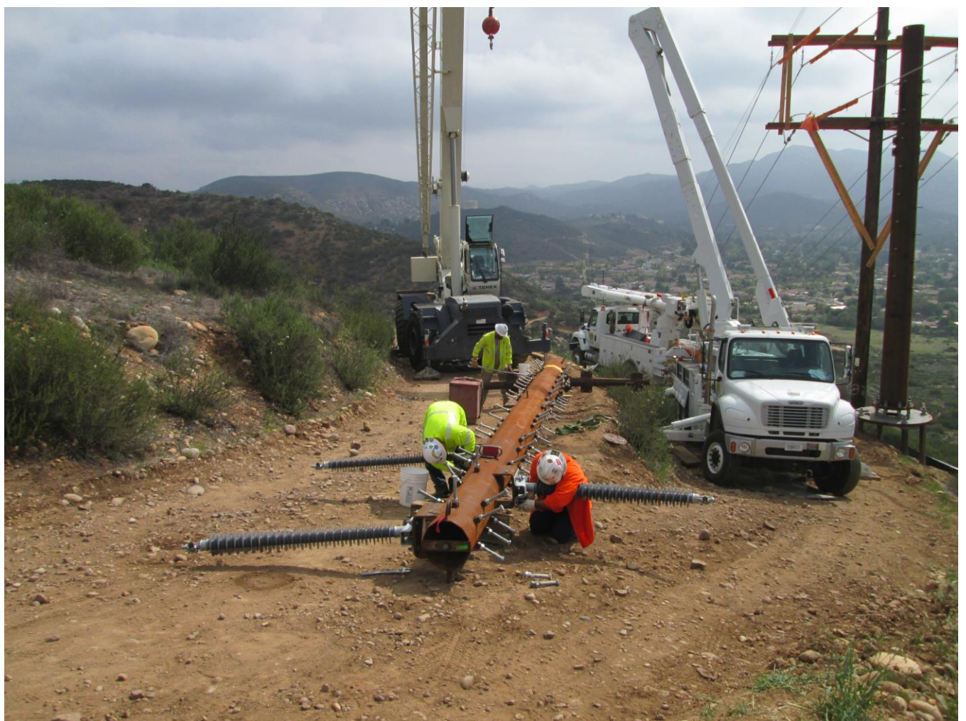
Photo 4: Construction crews were observed installing steel poles (above, Location 32). In accordance with MM-HAZ-2, visqueen was observed beneath staged equipment to prevent leaks/spills from being discharged into the soil.
