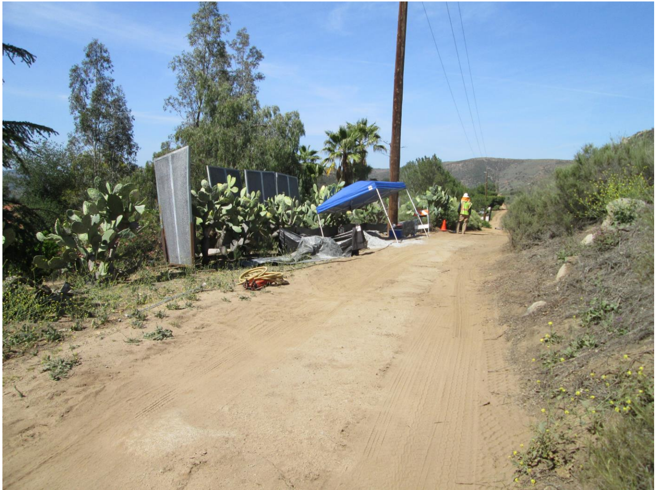
Photo 3: In accordance with MM-NOI-2, a noise barrier was observed being implemented adjacent to sensitive receptors (above, Location 56) during pole hole hand digging. Silt fencing on site was observed in good condition and functional in accordance with APM-HYD-1 and the Project SWPPP.
