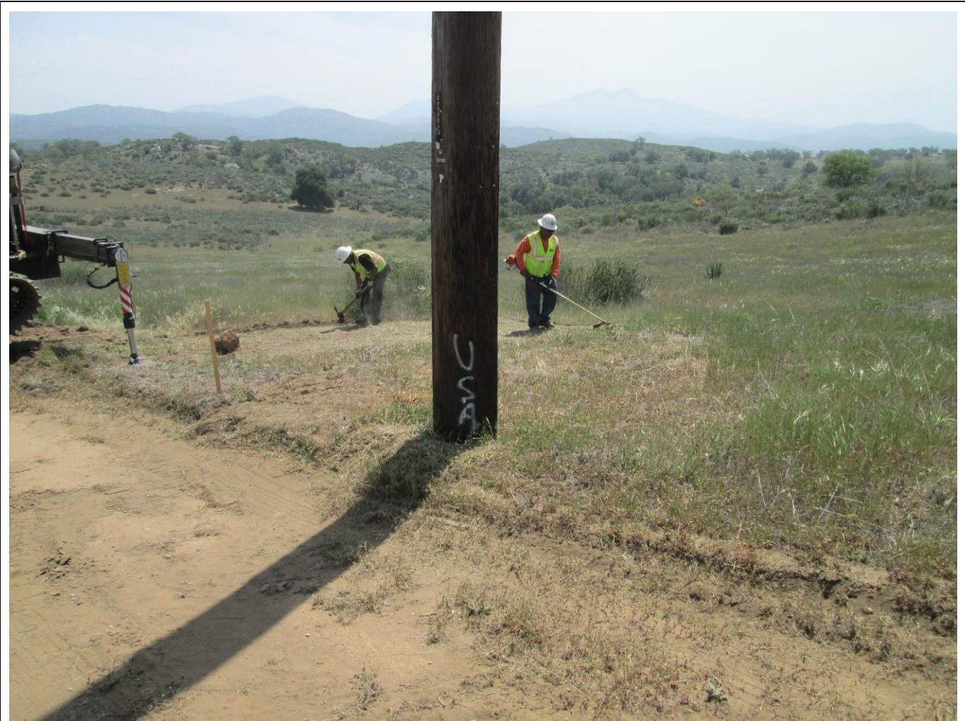
Photo 5: Construction crews were observed trimming vegetation at pole replacement work areas in accordance with APM-HAZ-2 and Project Fire Plan, and installing erosion control BMPs including silt fencing and/or straw wattles in accordance with APM-HYD-1 and the Project SWPPP (above, Location 97).
