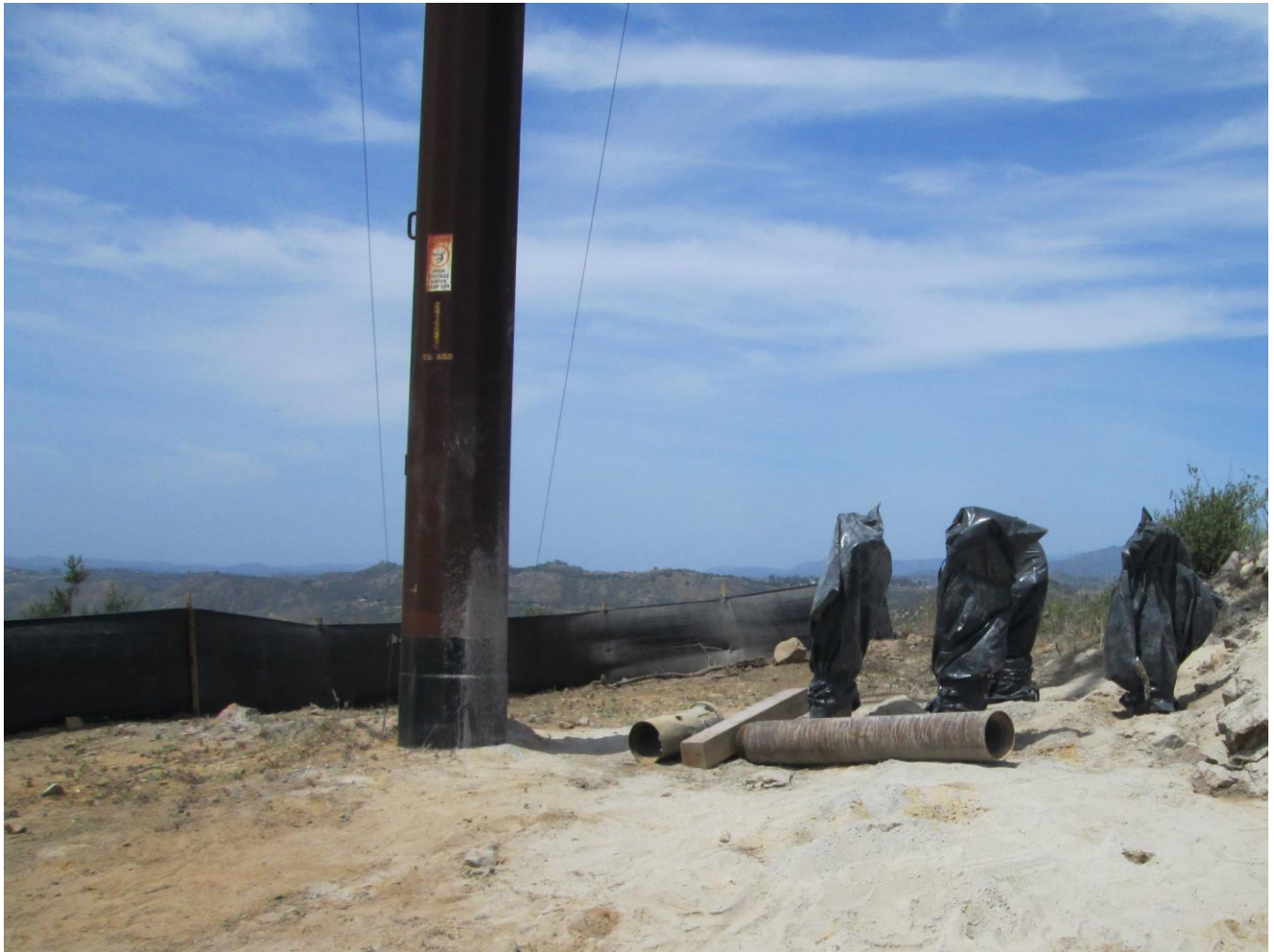
Photo 8: In accordance with MM-BIO-3, open holes and micropile foundations were covered to prevent wildlife entrapment.
