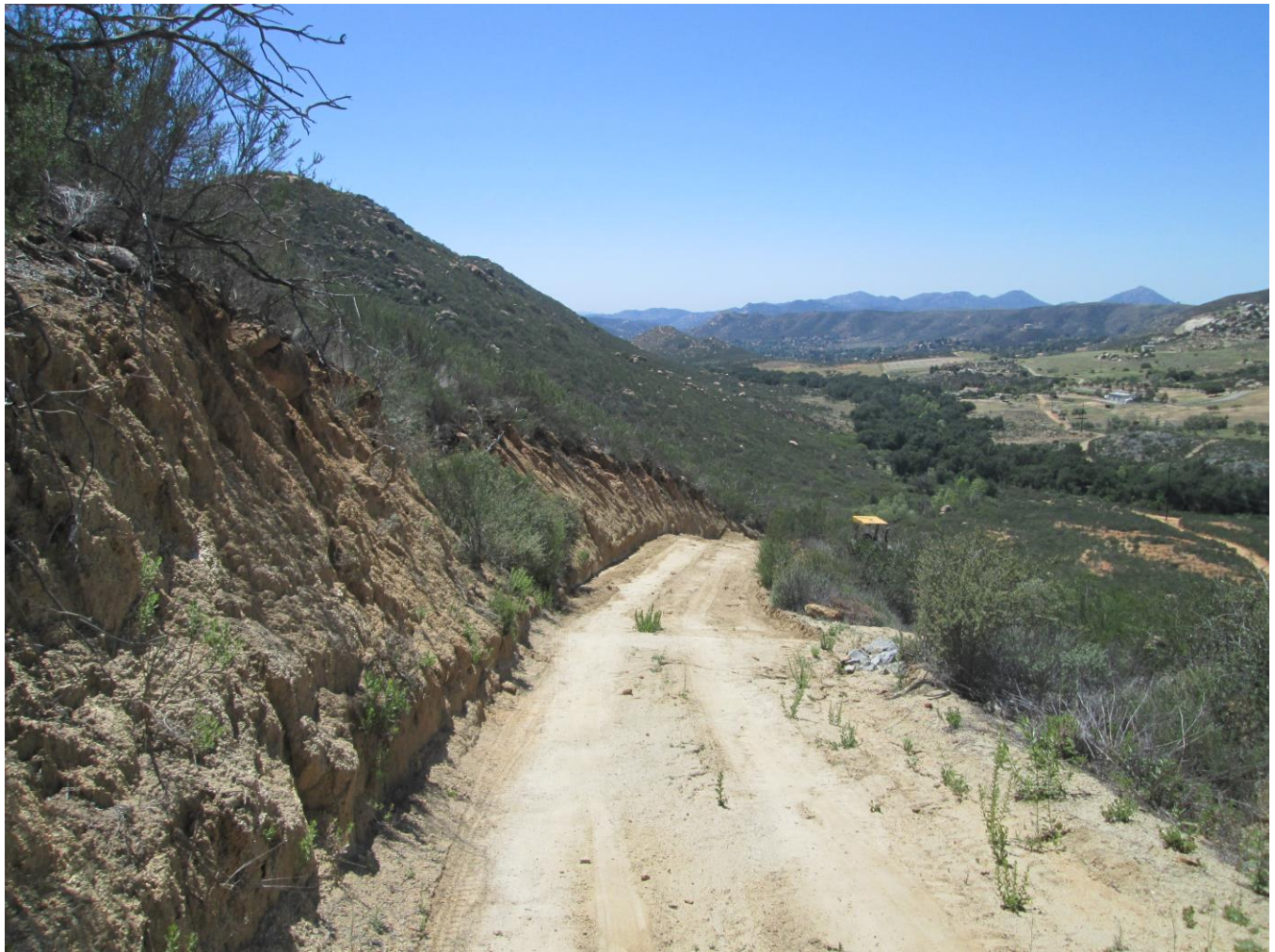
Photo 6: Construction crews were observed refreshing the main access road and maintaining existing water bars in accordance with APM-HYD-1 and Project SWPPP.
