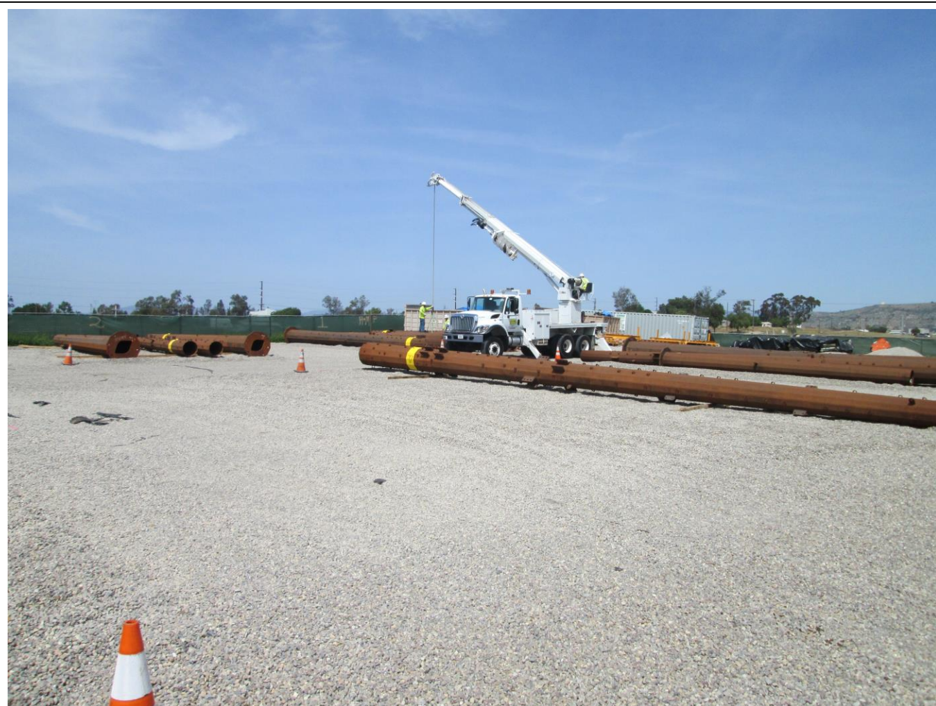
Photo 1: Delivery of steel poles and construction materials continued during the reporting period (above, Warnock Staging Yard). In accordance with APM-AES-1, the opaque mesh used as visual screening remains intact around the perimeter of the yard.
